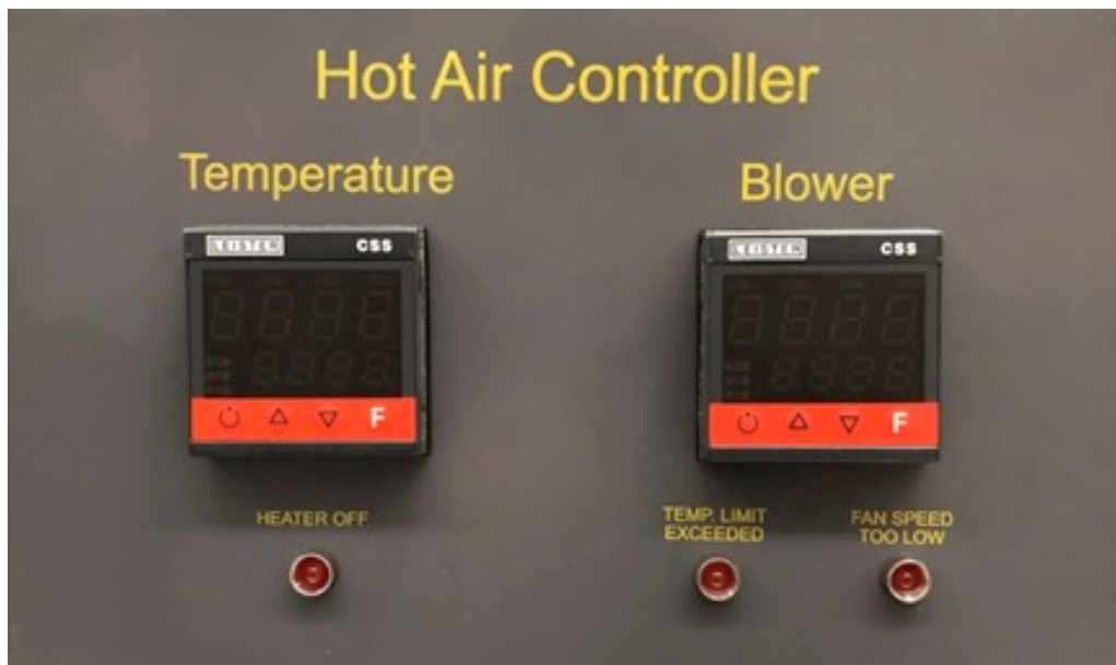
Fig. 1. Front face of a control box. Status LEDs are provided to indicate various fault states of the heat gun operation.
